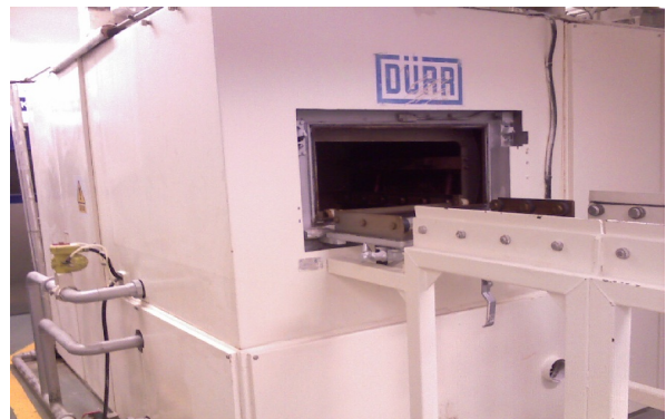
↑ Station de lavage
